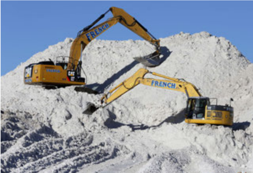
Framingham, Mass., officials overhauled their snow removal strategy by dividing the town into snow management zones based on geography and resources.
